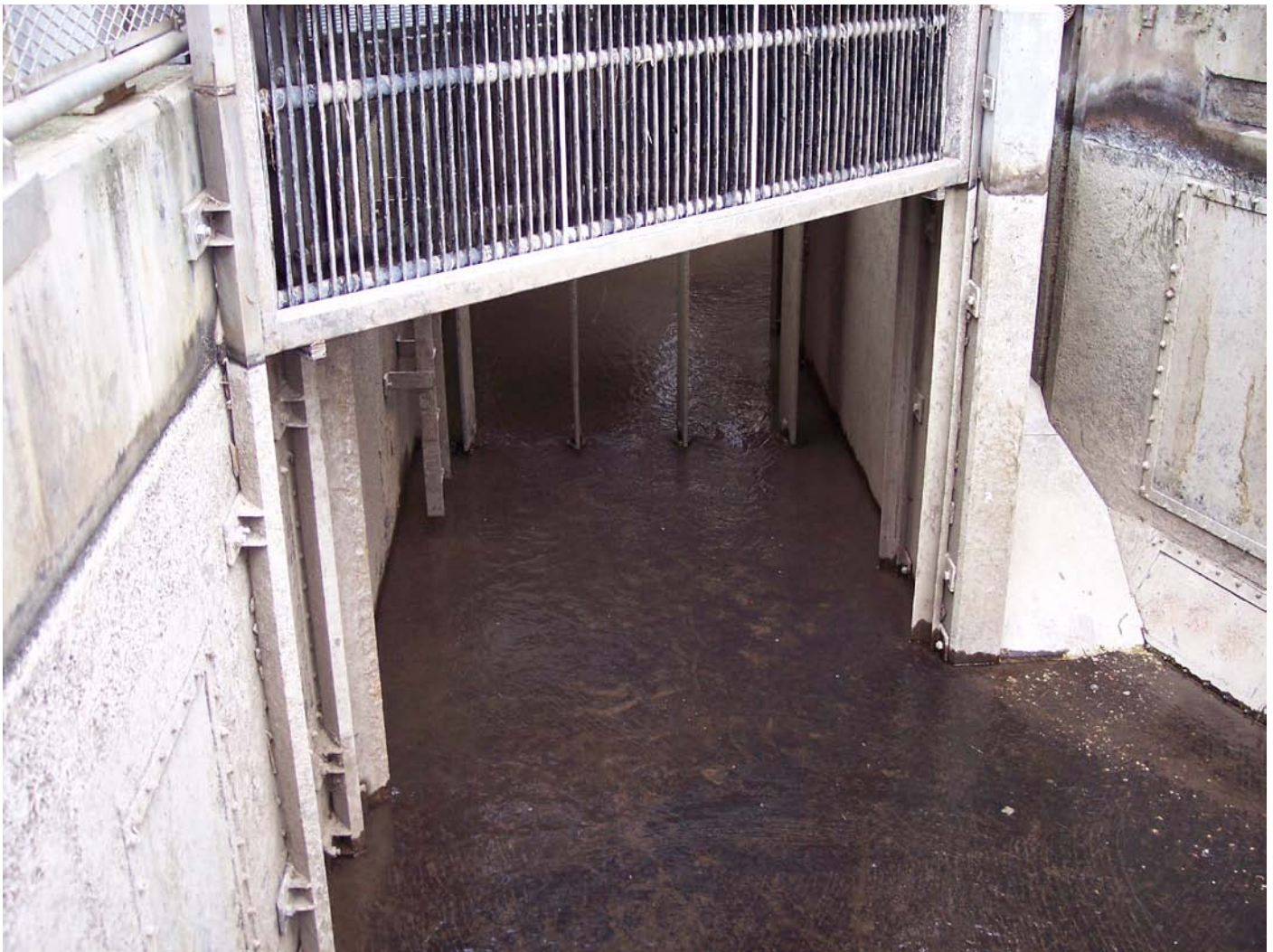
Figure 7 – North Shore Fish Ladder Counting Station Looking Upstream. Note the spacing on the channel bottom of the flow control vanes located behind the raised picketed lead panel and permanent blocking (1 ½ inch) welded to the bottom of the picketed lead frame at each end.
