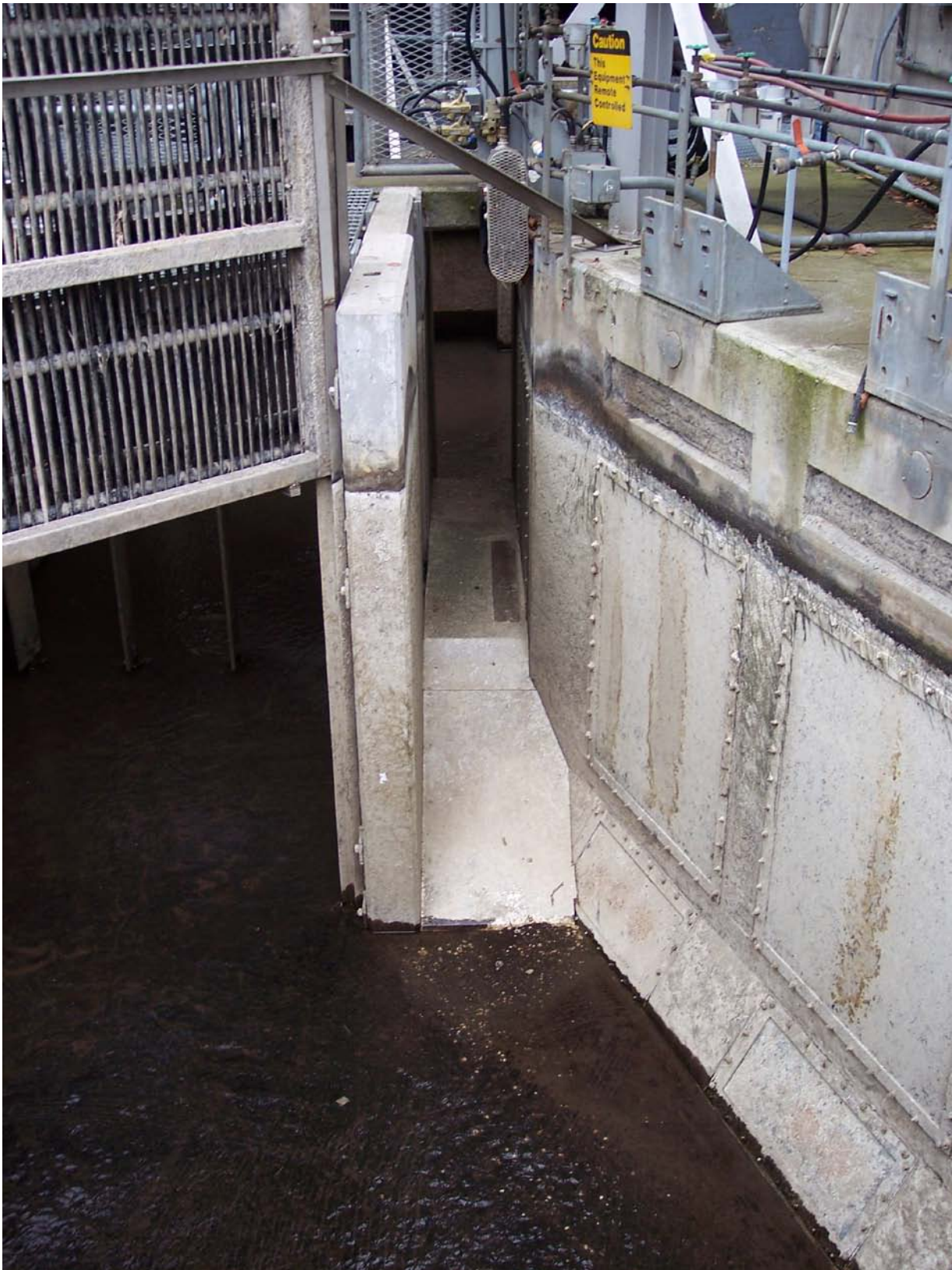
Figure 8 – North Shore Fish Ladder Counting Station Looking Upstream. Note the smooth plate ramps in lieu of grating on the approach to the counting slot.
