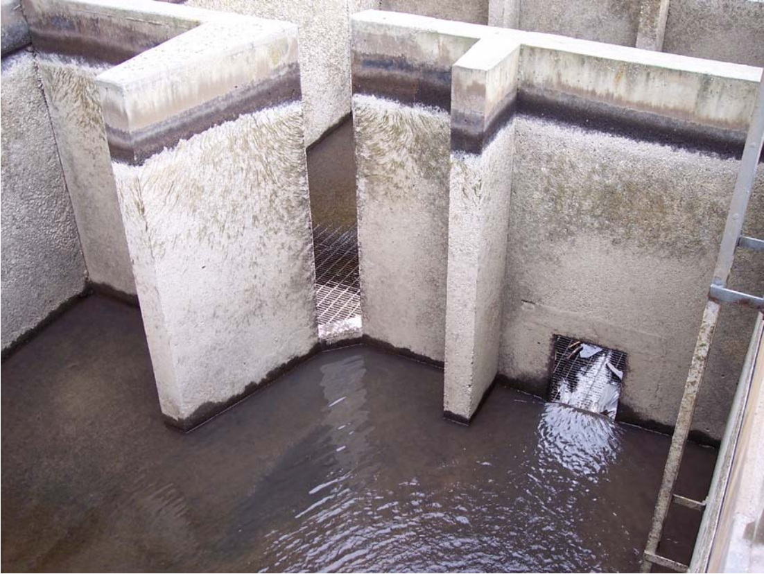
Figure 14 – North Shore Fish Ladder Control Section Weir 534 and Diffuser 6 Photo, Looking Downstream.
