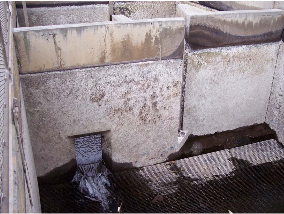
Figure 13 – North Shore Fish Ladder Control Section Weir 534 and Diffuser 6 Photo, Looking Upstream.
